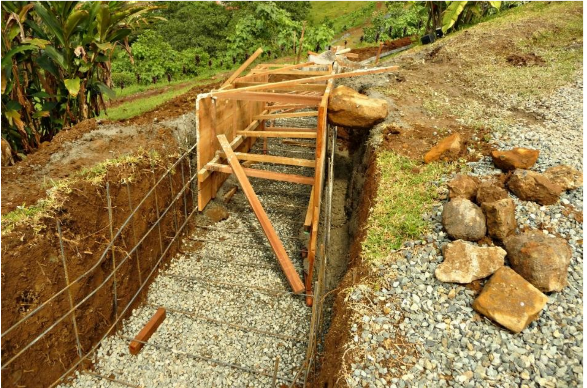
In order to conquer the steep dropoff, a trench needed to be dug.
