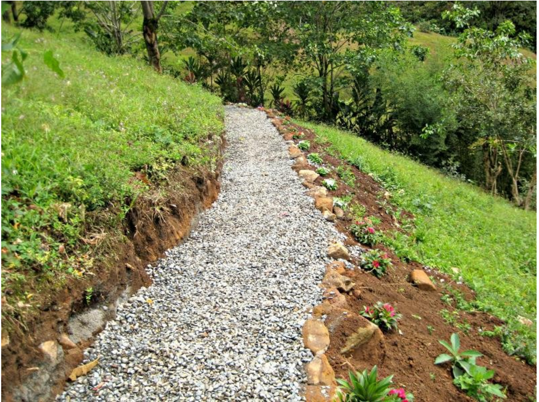
The south sendero is made of layers of sand, stone and cement, lightly watered.
