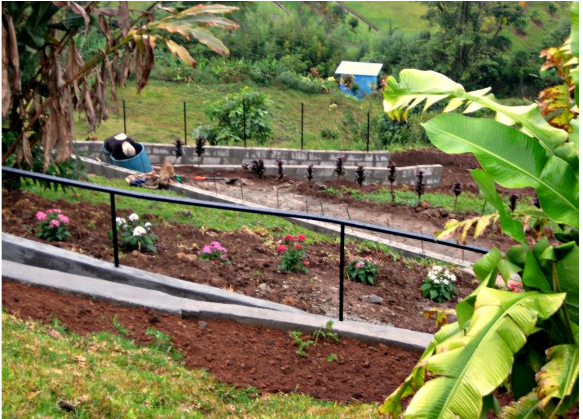
Retaining walls were constructed, mostly of concrete block, starting from the top.
